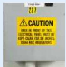
Hazard warning signs
