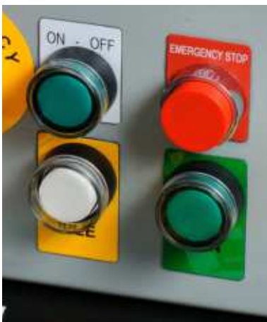
Control panel labels
