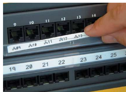
Punch block & patch panel labels
